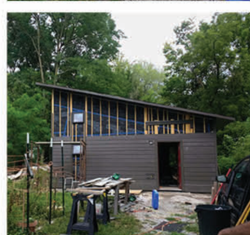
PROGRESS OVER TIME. AFTER THE ADU'S EXTERIOR WAS COMPLETE, WORK BEGAN INSIDE ON STRAW BALE INSTALLATION AND PLASTERING. PHOTOS COURTESY OF ADRIENNE STOLWYK.
