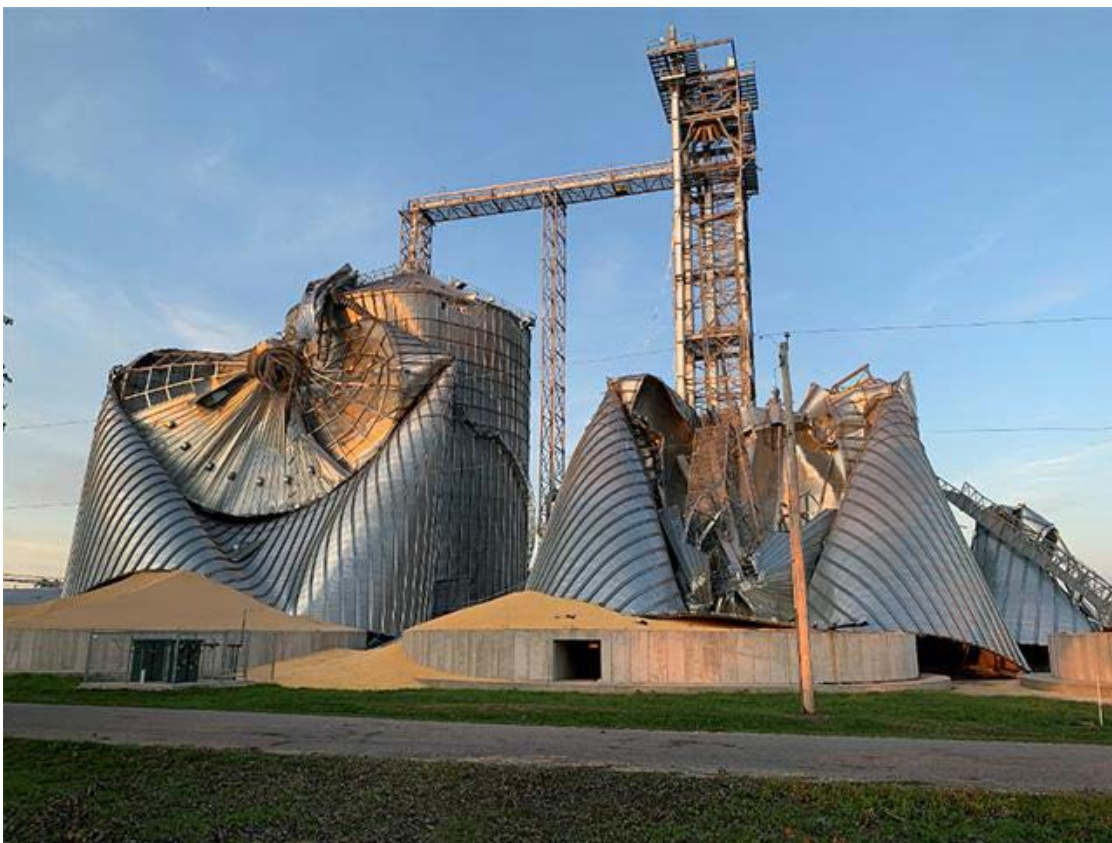
DERECHO DAMAGE AT THE HEARTLAND CO-OP IN LUTHER, IOWA. PHOTO BY TODD HULTMAN FOR DTN Progressive Farmer
